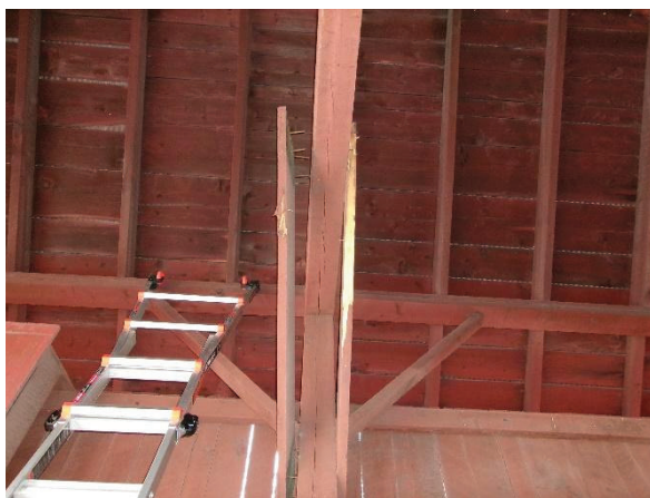
Broken Connection at Crossbeam and Knee Brace
