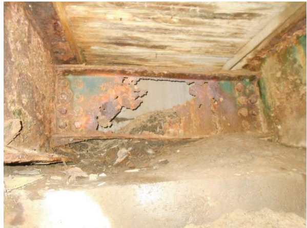
100% Section Loss in Diaphragm
